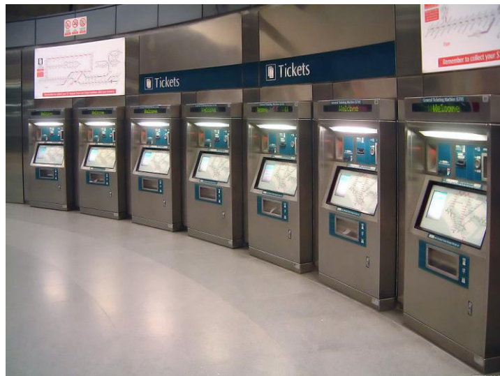
Automated Fare Collection Systems
